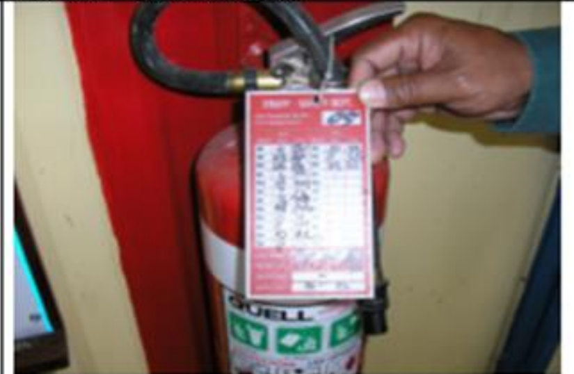
Fire extinguisher last checked in March this year in an area where control of flammable substances is poor.
