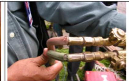
Hoses of Oxygen/acetylene gas welding in very poor condition – potential fatality
