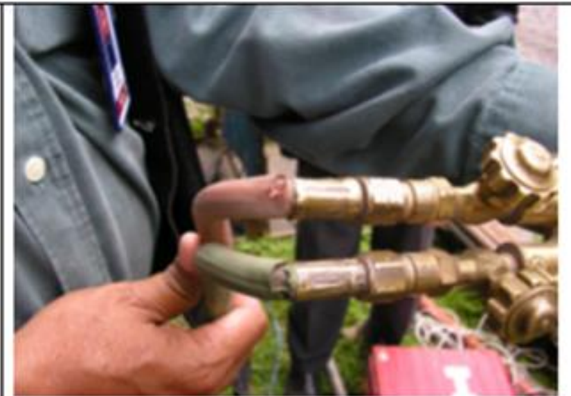
Hoses of Oxygen/acetylene gas welding in very poor condition – potential fatality
