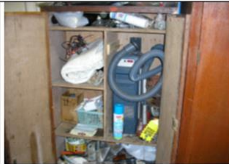
Poor housekeeping and control of flammable substances
