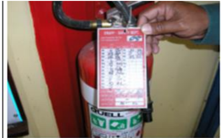
Fire extinguisher last checked in March this year in an area where control of flammable substances is poor.
