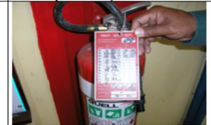
Fire extinguisher last checked in March this year in an area where control of flammable substances is poor.
